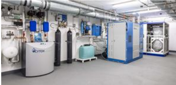
Image 3: CYTOK's reference plant at the Bernsteinsee holiday and leisure resort (Lower Saxony) with electrolyzer and methanation unit
